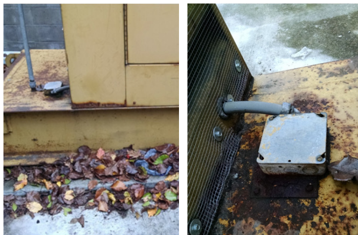
A single-wall tank and the level sender electrical box is exposed to the weather. Water is getting into the tank.
